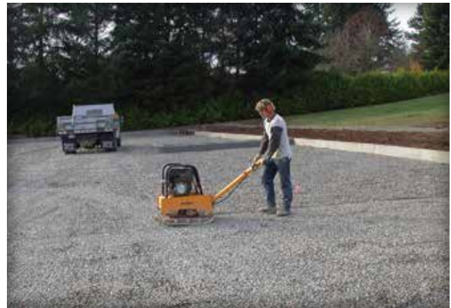
Figure 22. A 13,500 (60 kN) vibratory plate compactor is used on this ASTM No. 57 stone base.
