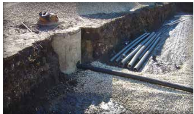
Figure 8. Partial infiltration designs typically use perforated pipes raised above the soil subgrade. This enables capture and infiltration of some runoff.
