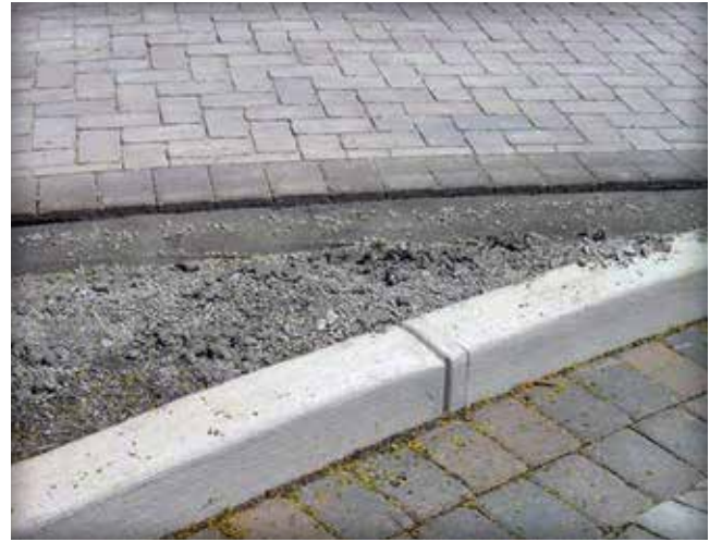
Figure 20. A PICP walk with a troweled concrete toe sits next to a driveway with a formed and cast-in-place concrete curb. Concrete toes should only be used for pedestrian applications.
