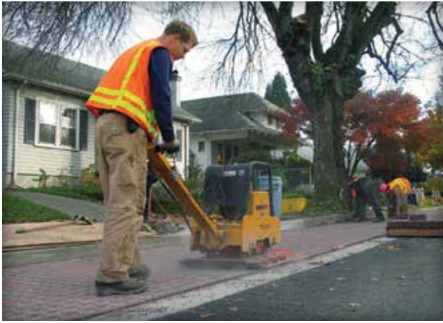
Figure 30. PICP paver compaction shows that pavers need to be set about \frac{3}{4} in. (19 mm) above their final elevation before compaction and \frac{3}{8} in. (10mm) after compaction to account for downward movement.
