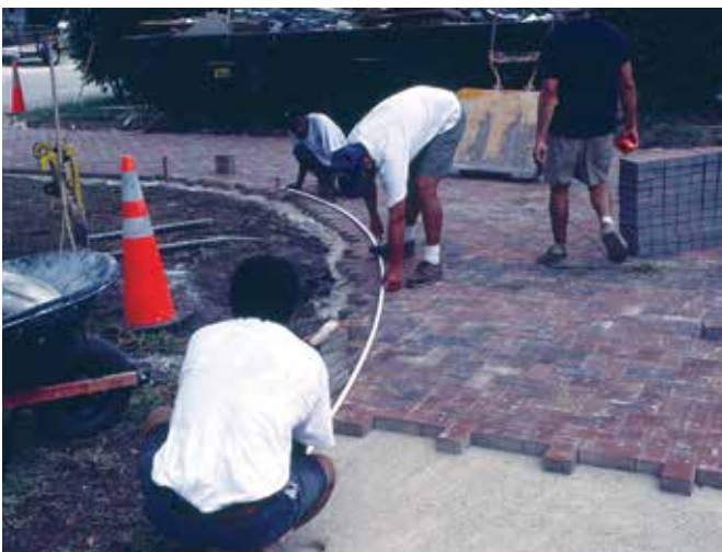
Figure 13. Marking pavers for saw cutting. The cut pavers are carefully removed and edging is placed against the pavers.
